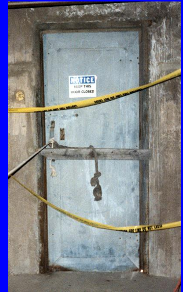
Locked and blocked exit
